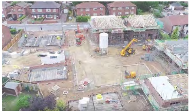
Drone footage of progress at Byram where Selby DC are building 13 new council homes for affordable rent funded by Homes England
